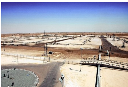
Pipes carry steam to the oil field, where it is injected underground, thinning the heavy oil for pumping
